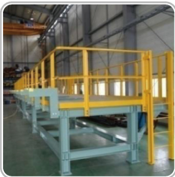
Pipe Rack Unit
