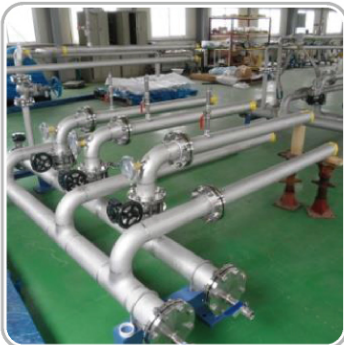
Machine Unit Pipe
