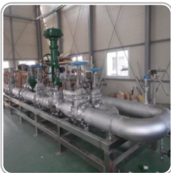
Flow Meter Unit
